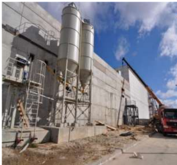
Fig. 10. Arrangement of the storage bunker for cementation facility outside the CRWP building
