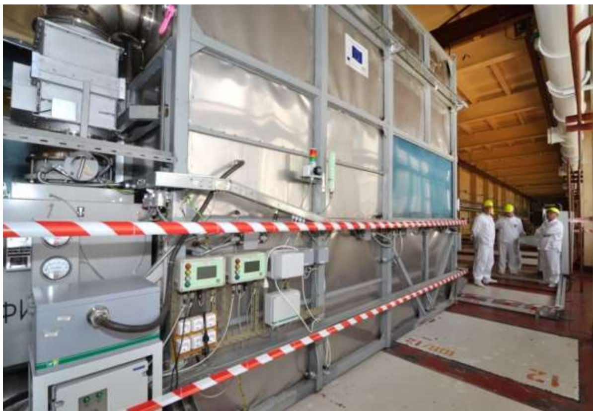
Fig. 3 Arrangement of the SRW extraction installation in the storage facility of auxiliary building-1.
