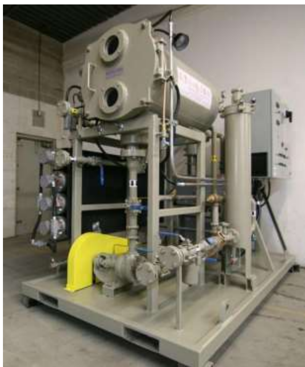
Fig. 8. View of the oil purification installation
